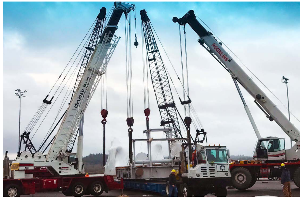
Local contractor Rognlin's, Inc. used four cranes to lift a record heavy piece of over-high, over-wide equipment at Terminal 4 last month.
